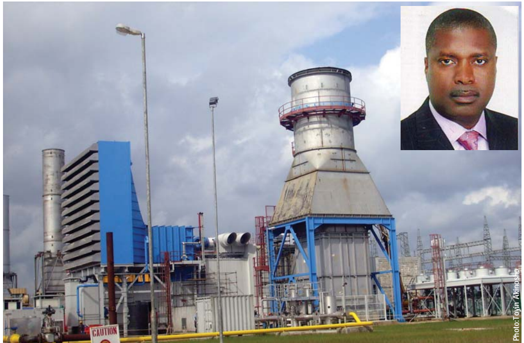
The generation part of the Ibom Power Plant is ready. On the foreground, in yellow, is the gas line. Inset is Obong Nsima Ekere, who is chairman of the boards of the Ibom power company and the Akwa Ibom Investment and Industrial Promotion Council (AKIIPOC), the investment arm of Akwa Ibom State Government
